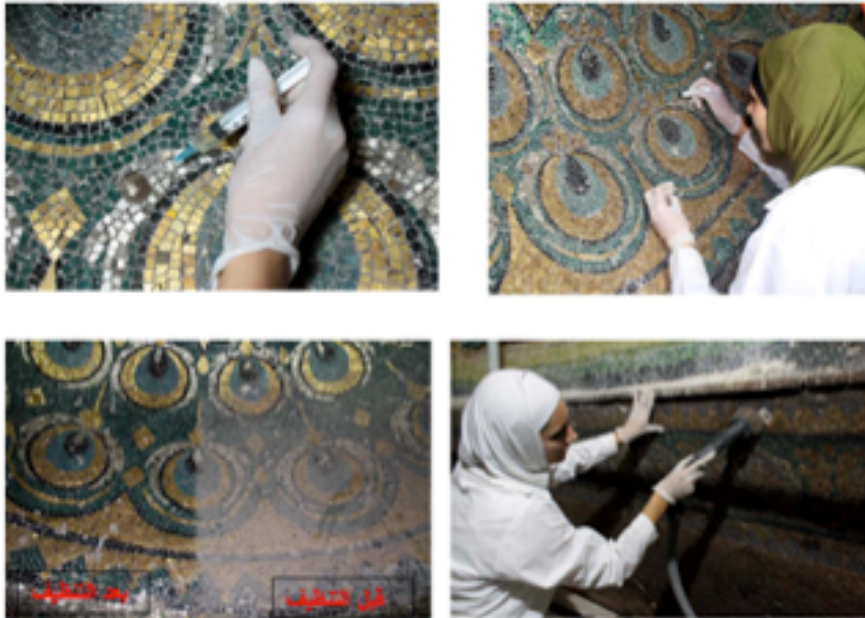
Hashemite restoration of the mosaics in the Dome of the Rock in 2015
